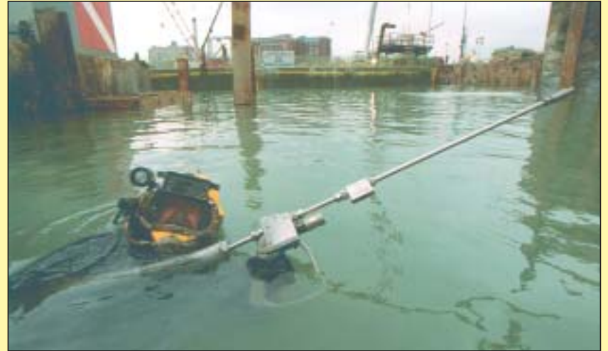
A diver with Hennigan Engineering Hydrolasing equipment by Jetstream of Houston descends into Boston Harbor to remove concrete overpours on a tunnel foundation, as part of Boston's "Big Dig" Central Artery/Tunnel project. (Photo courtesy of Boston Globe)
