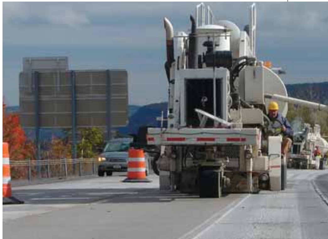
Diamond grinding is applied to I-88 near Albany, N.Y. Photo credit: IGGA
