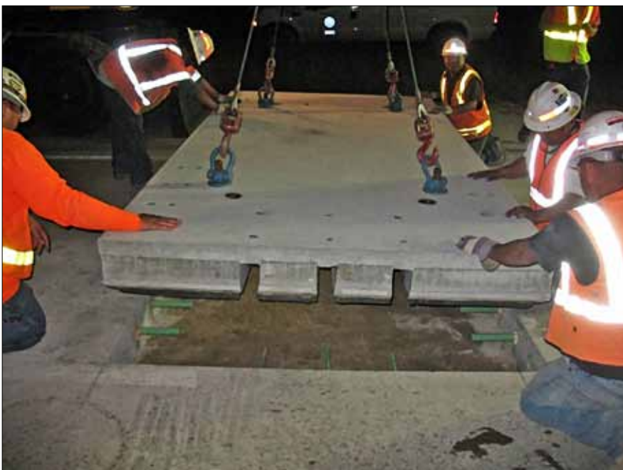
◀ Precast concrete pavement slab is lowered into Utah's I-15 between Clearfield and Layton.
