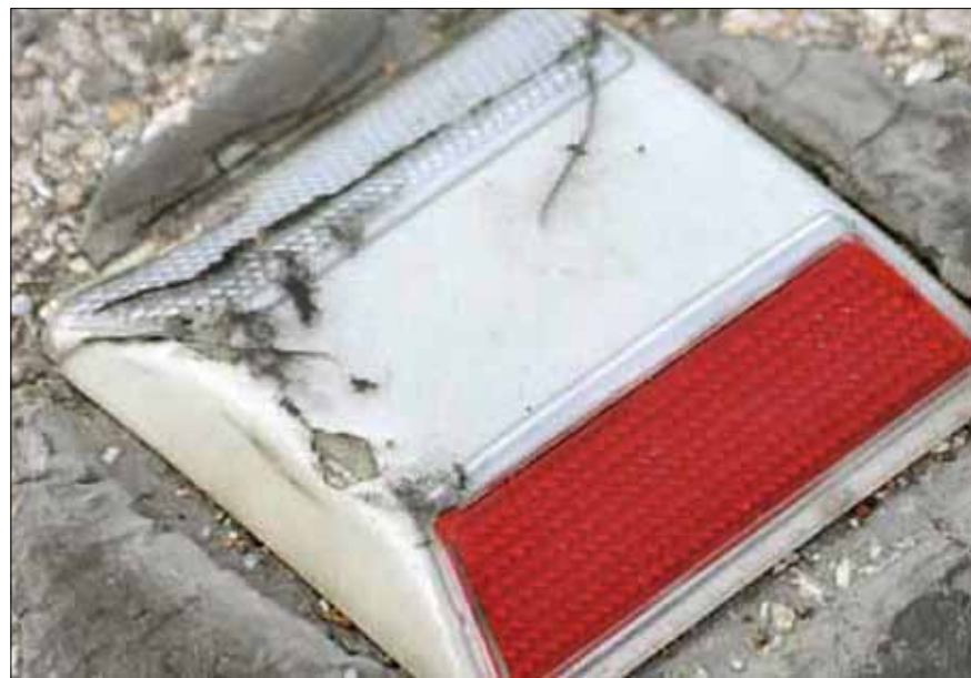
▲ Damage to shell of retro-reflective raised pavement marker could be caused by something as simple as a stone wedged in tire tread.
