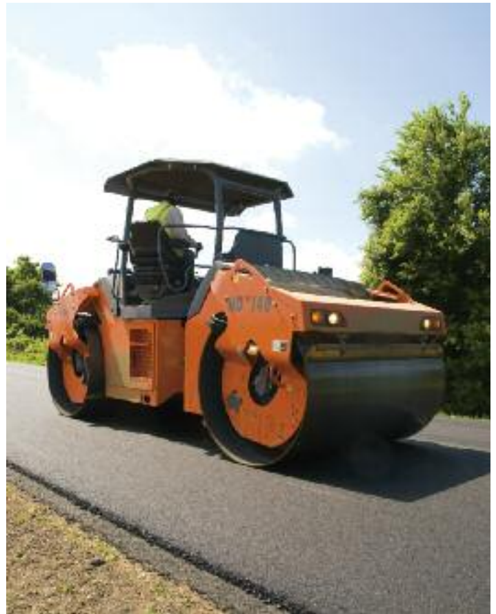
HD+ 140 VV, among the first in North America, compacts in northeast Louisiana
