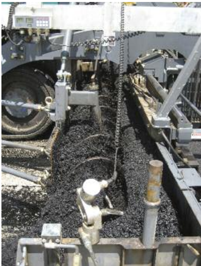
Careful set up of screed extensions and internals critical to achieving IRI of below 40 in. per mile, resulting in 97 percent of smoothness bonus for contractor
