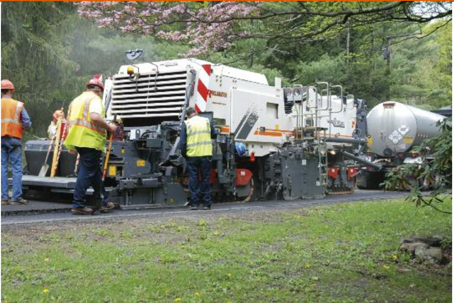
U.S. Contractor Reclamation Inc. foamed asphalt-recycles Zena Road in New York State adjacent to Catskills State Park
