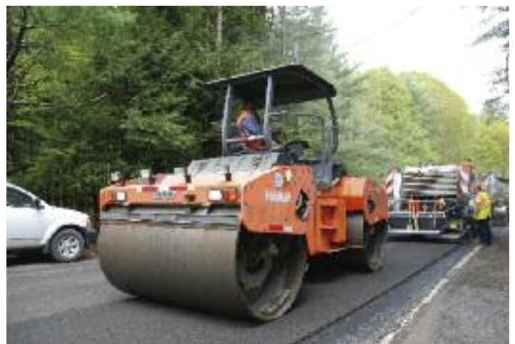
Hamm HD 130 HV 84-in double-drum steel vibratory roller was one of three compactors on foamed asphalt mix
