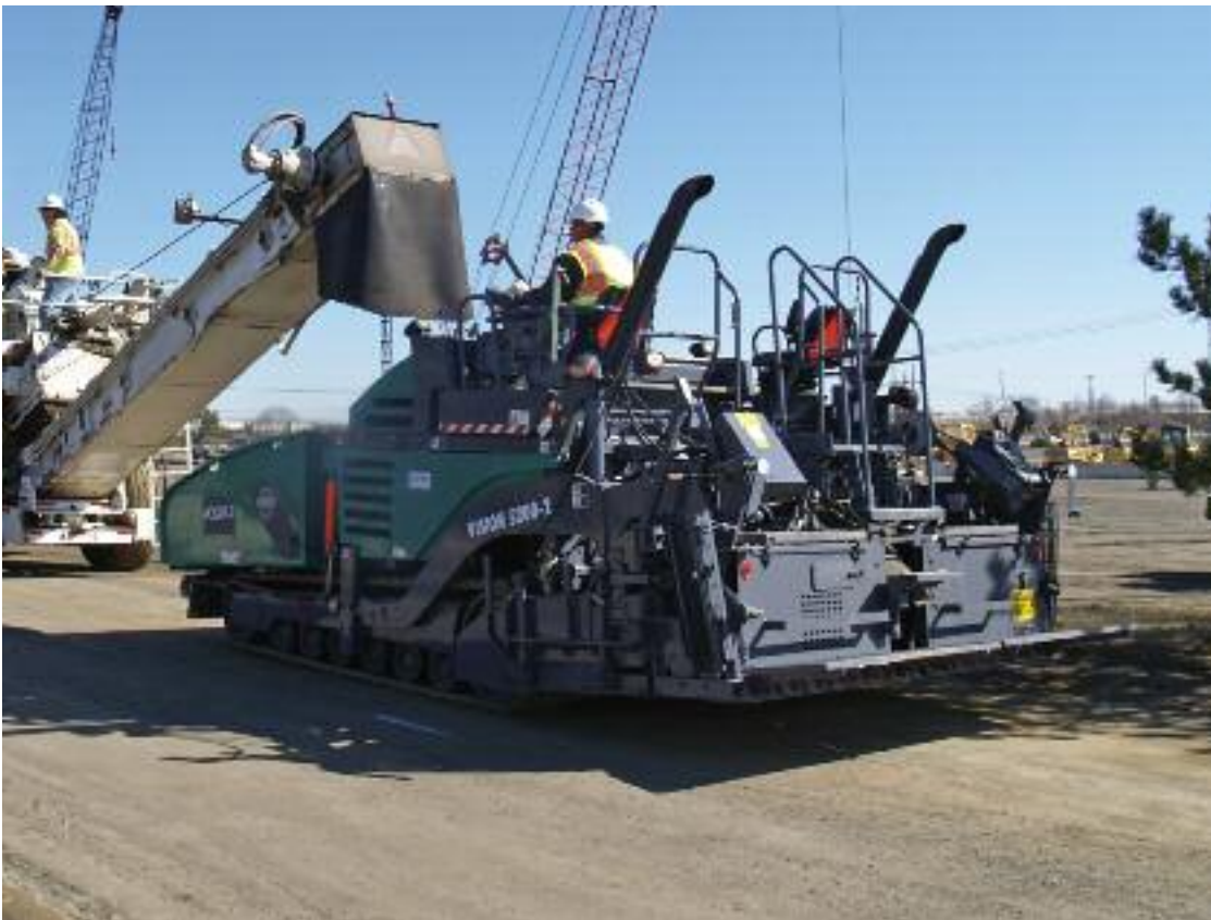
◀ Vögele Vision 5200-2 and material transfer vehicle get ‘dry run’ at Local 825 training facility; training also included planing with a Wirtgen W 2100 cold mill
