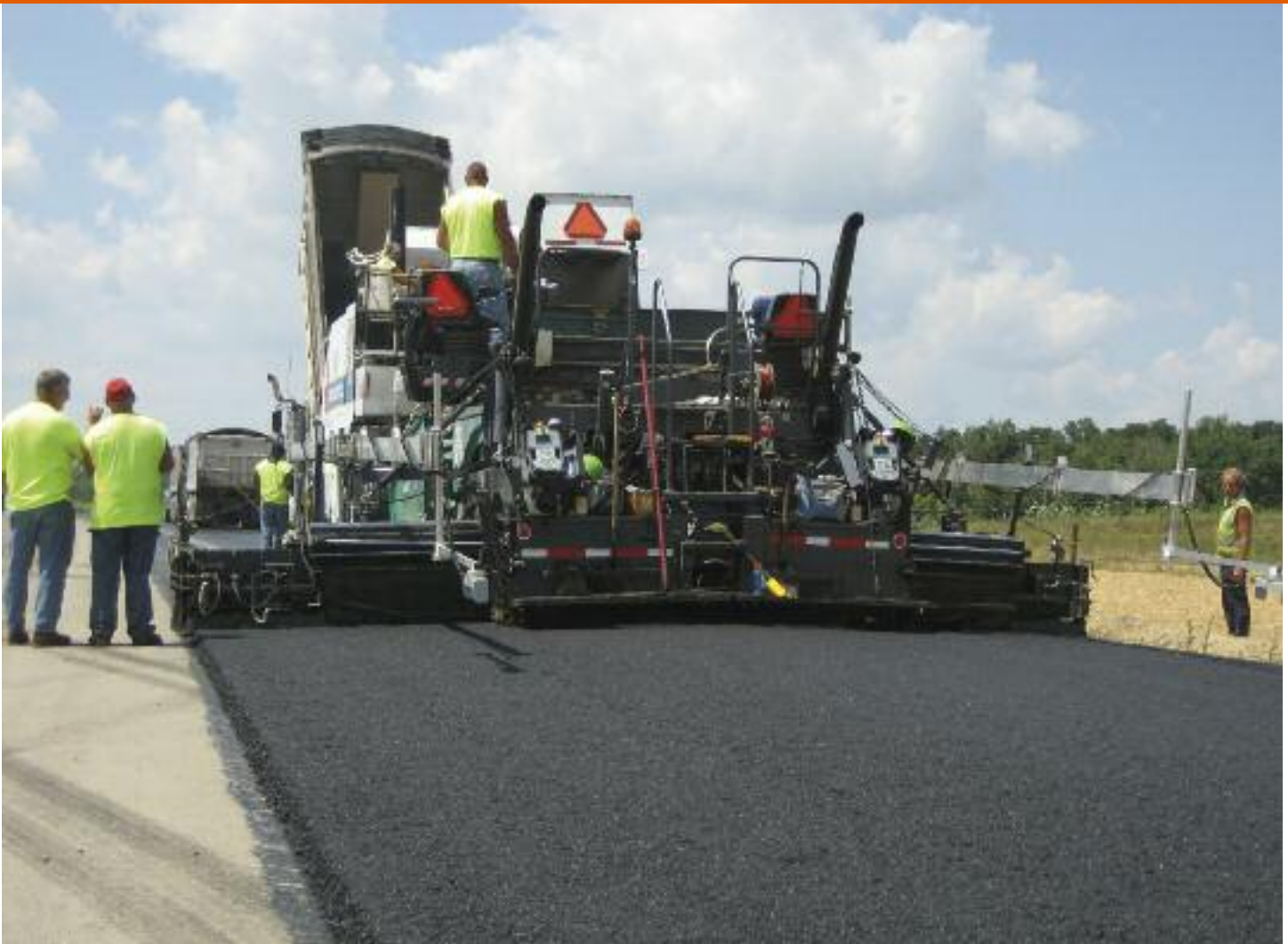
Paving in full 23-ft.-wide pull enabled Shelly & Sands to place pavement in one width without longitudinal joint, improving long-term durability of pavement under seven-year warranty
