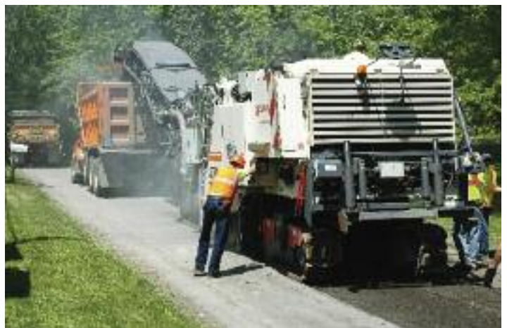
With conveyor mounted, Reclamation Inc. cold mills pavement with Model 2200 CR from Wirtgen Group
