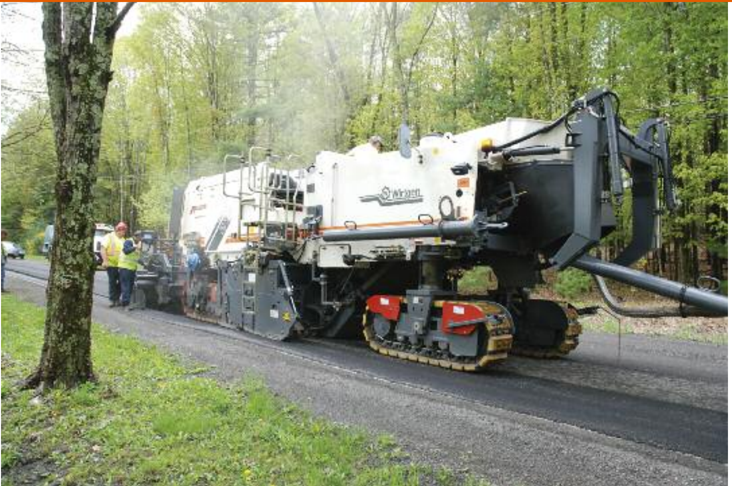
With conveyor removed, Wirtgen 2200 CR recycles pavement surface in-place, but also can cold-mill pavements with conveyor mounted
