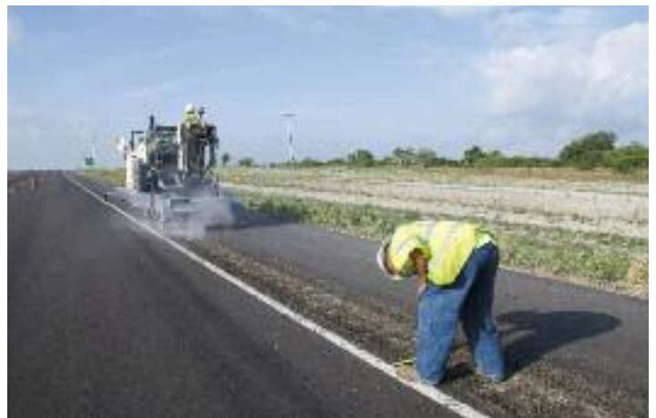
PennTex personnel check cut depth of fresh rumble strips on U.S. 77 north of Victoria, Tex.
