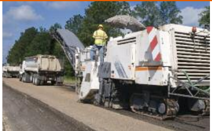
On different U.S. 165 project, Gilchrist's W 2200-12 cuts asphalt off concrete underlayment a full-lane wide, prior to percussive demolition
