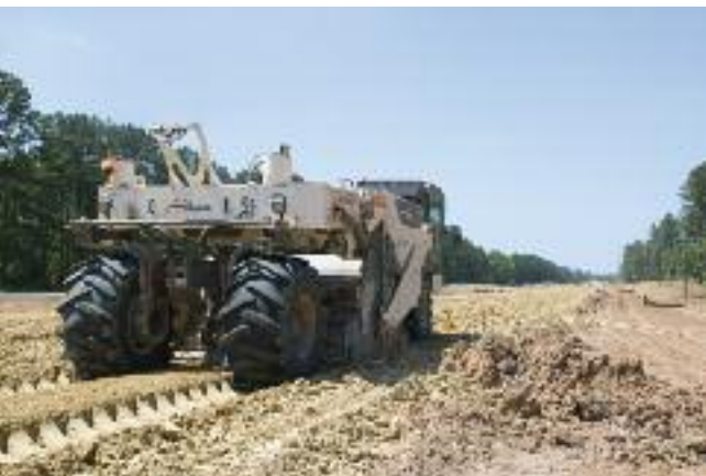
One of five WR 2400s of Gilchrist Construction turns over base material to remove excess moisture in ROW of reconstructed U.S. 167 in central Louisiana
